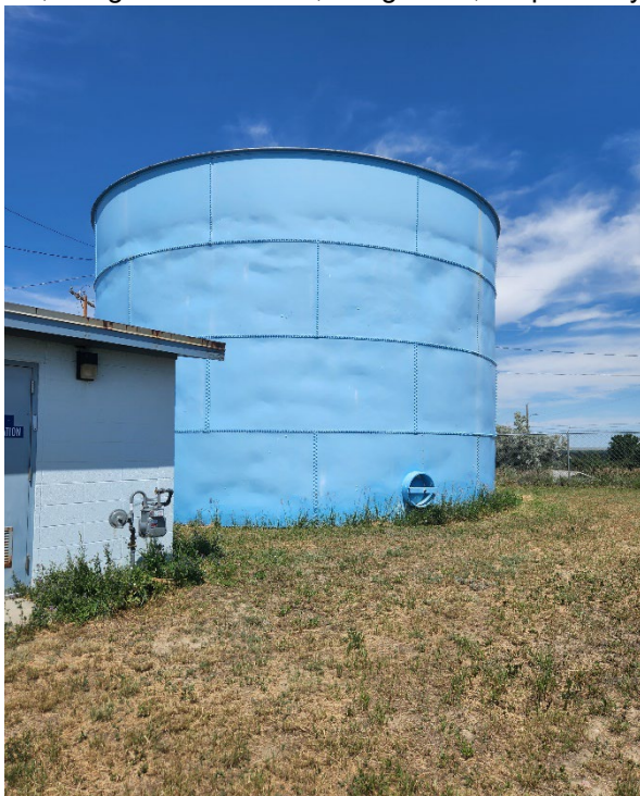
Figure 6 - 176,000 gallon water storage tank
