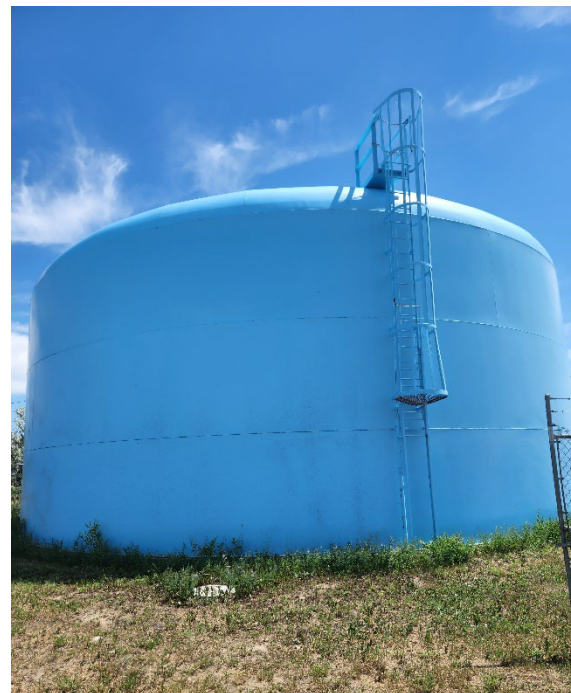
Figure 7 - 400,000 gallon water storage tank
