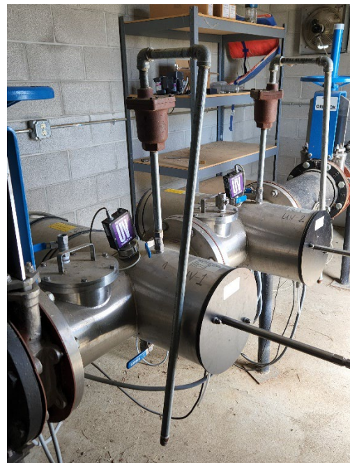
Figure 4 – Ultraviolet Treatment Units
